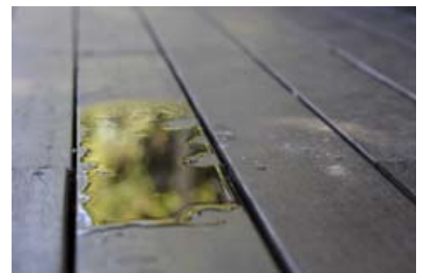
Water left on timber can cause fixings to deteriorate and rust
