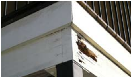
Check bearers and joists for warping or cracking
