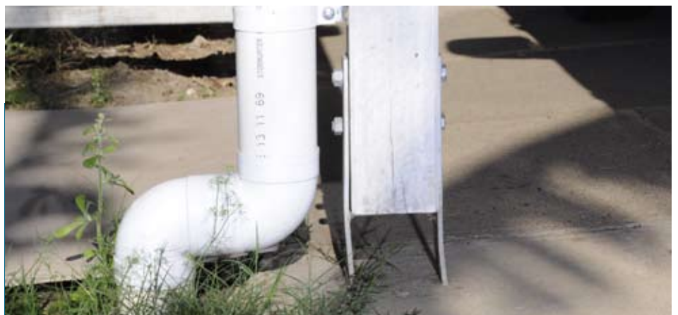
Inspect post brackets for bending or stressing
